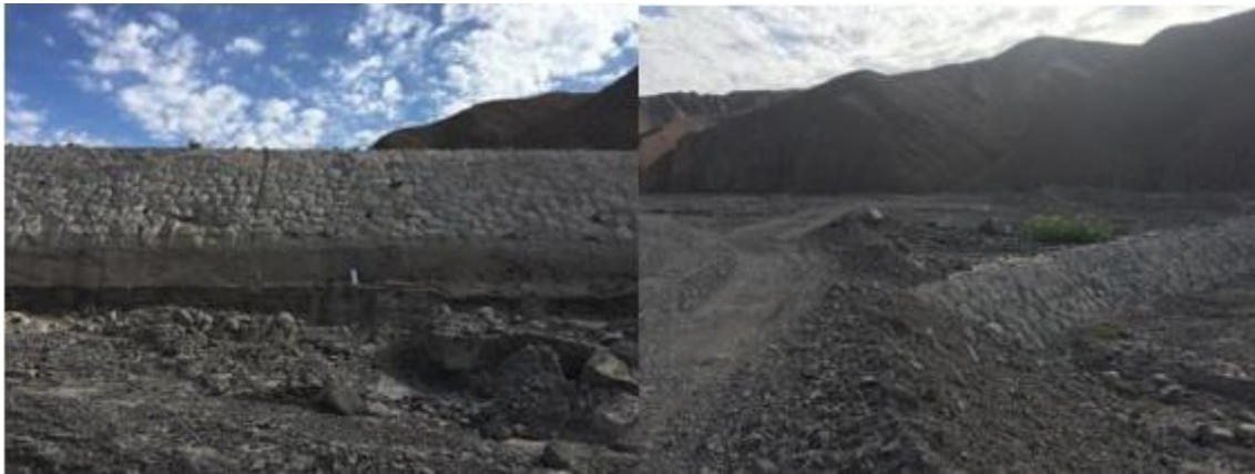
Figure 12. Left: View from Dike 1 downstream, where foundation undermining is shown below dam foundation and its dissipation pool after the debris flow of 2019. Right: The vessel of the dam clogged with solids by debris flow of 2019.
