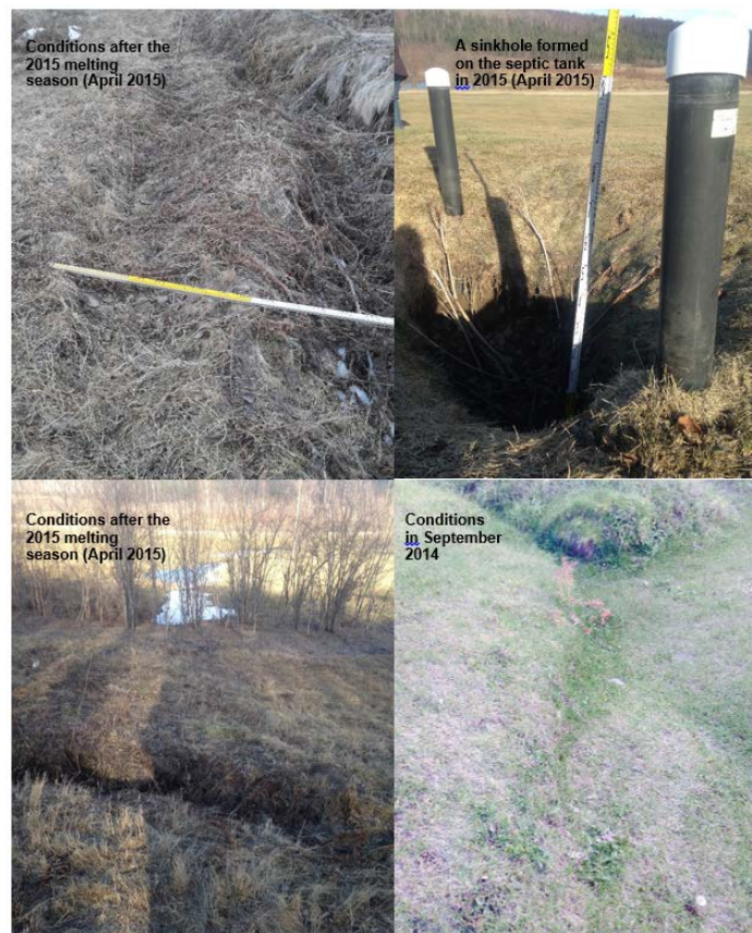
Figure 7. Subsidence and topographic changes observed at Bob and Mary Martin's property.
