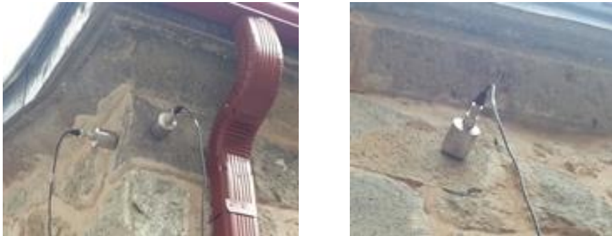
Fig. 12. Some images of the measurements of Molla Siyah Mosque after the restoration
