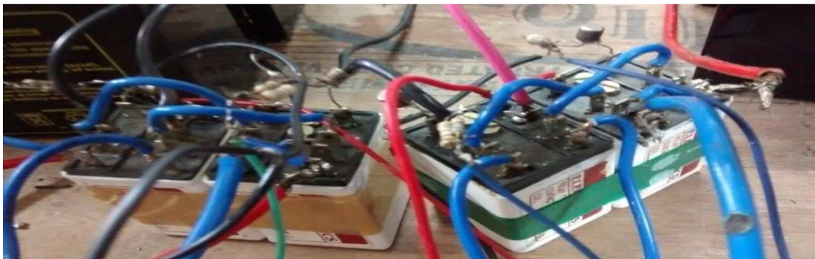
Fig. 5 Four Relays are connected to two Motors
