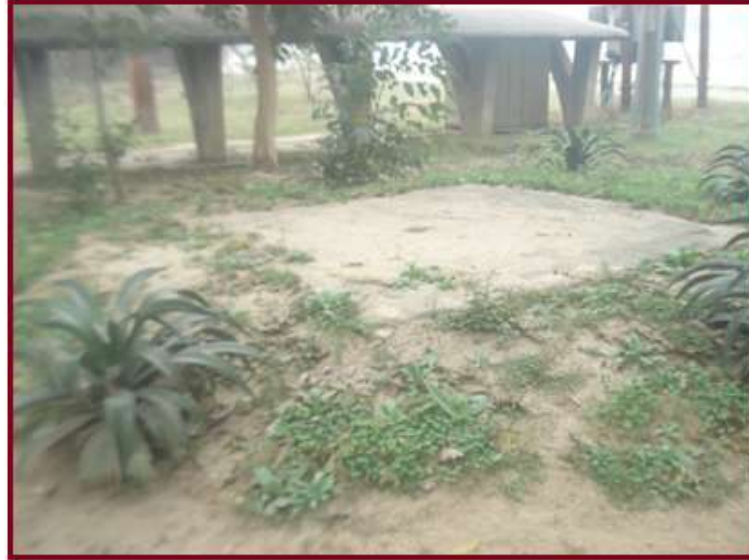
Fig.16. Well of the west wing of the MAO collage is covered by concrete.
