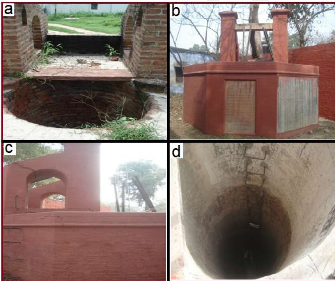
Fig. 15. Earlier image of wells in the east wing of MAO College their present condition, developed cracks and inside images of the wells
