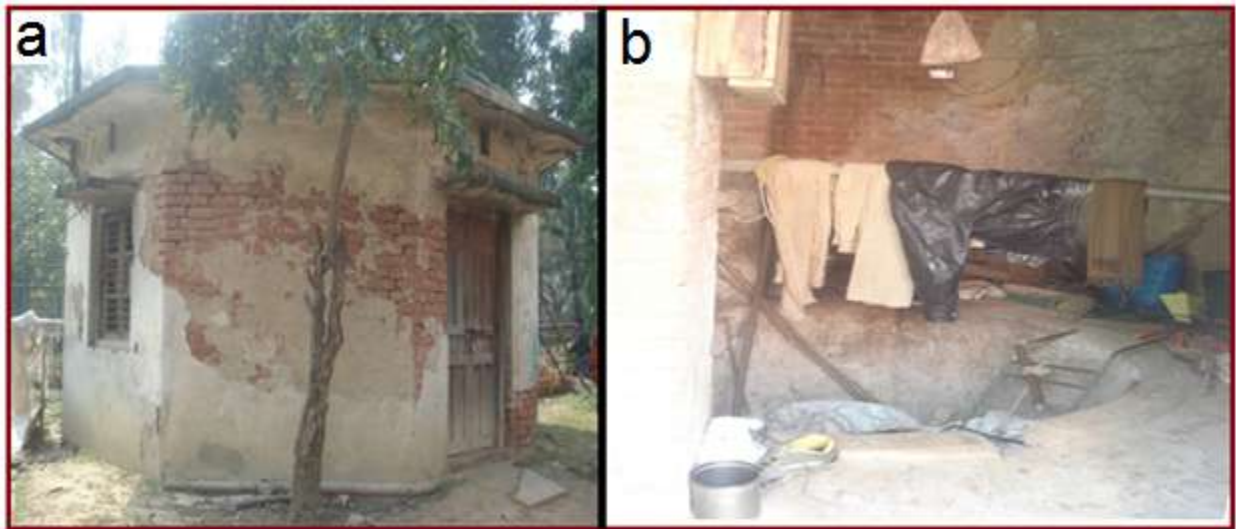
Fig.17. Well in front of Victoria gate is covered inside the room and their bad condition
