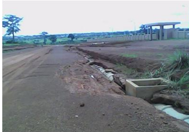
Figure 2. Picture illustrating the destruction of road shoulders by raining water and soil erosion
