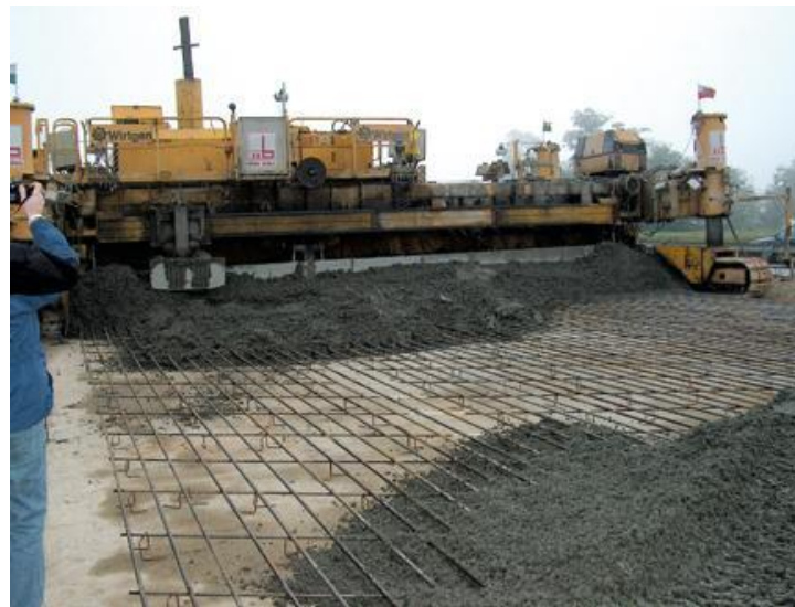
Fig. 2. The works conducted during the construction of a continuously reinforced concrete highway
