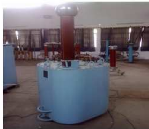
Fig. 3 High voltage Testing transformer
