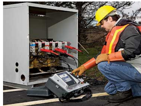
Fig.1. Linemen trying to measure the various parameters of the transformer.
