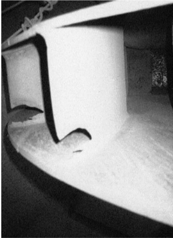
FIG 3. EROSION OF WINGS OF ID FAN
