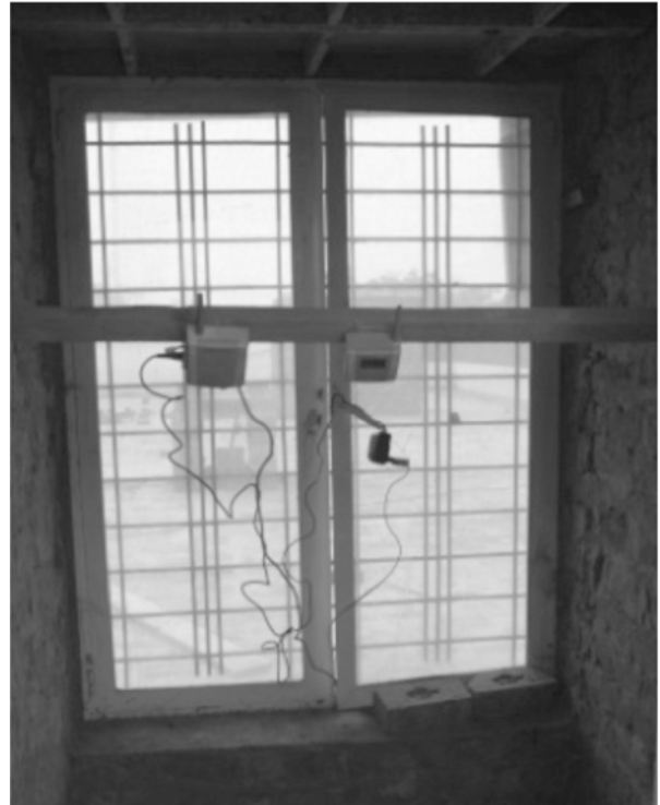
FIG. 6(a). PROBE INSTALLED
