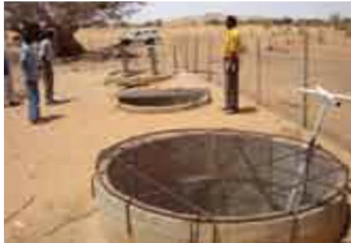
Figure 1. Improved Hafir with Two filtration Wells in North Kordofan (UNICEF ,2009)
