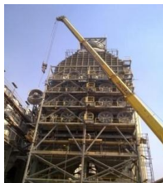
Fig.21: Heat Exchanger before FF at Cooler area.
