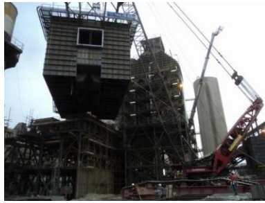
Fig.23: Fabric Filter is lifted up on its way to take the Gravel Bed Filter place.
