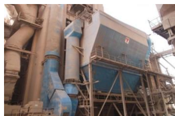
Fig.15: The converted bypass filter after conversion into FF in Tourah cement Co. (December 2011).
