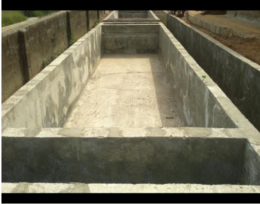
Figure 3(a). Reinforced Concrete Cell
