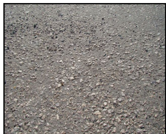
Fig. 5. Aggregates loss on Rick Turner Road.
