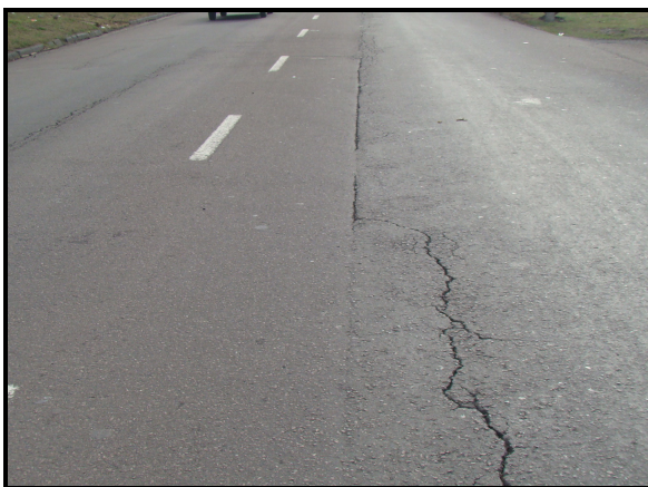
Fig. 3. Longitudinal and crocodile cracks on South Coast Road
