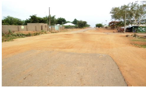
Plate 3: Wears and tears of road materials and no side drainage, on Taraba Road minor road.
