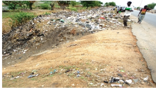
Plate 8: Road shoulder breakage and illegal waste collection point along Mubi Bye-Pass major road.
