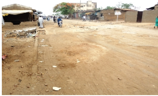
Plate 7: Blocked drains, and wears and tears of road materials on Taura minor road.
