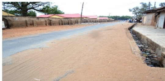
Plate 5: Wears and tears of road materials with an unsightly side drainage on Benjiram minor road.
