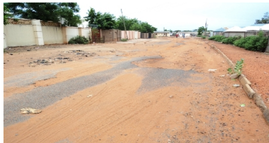
Plate 4: Wears and tears of road materials and no side drainage on Bole Street minor road.
