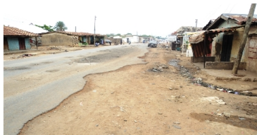
Plate 6: No sides drainage and worn out road materials in Midili Street minor road
