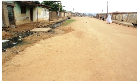
Plate 1: Aliya Street earth road with inadequate sides-drain on a minor road.
