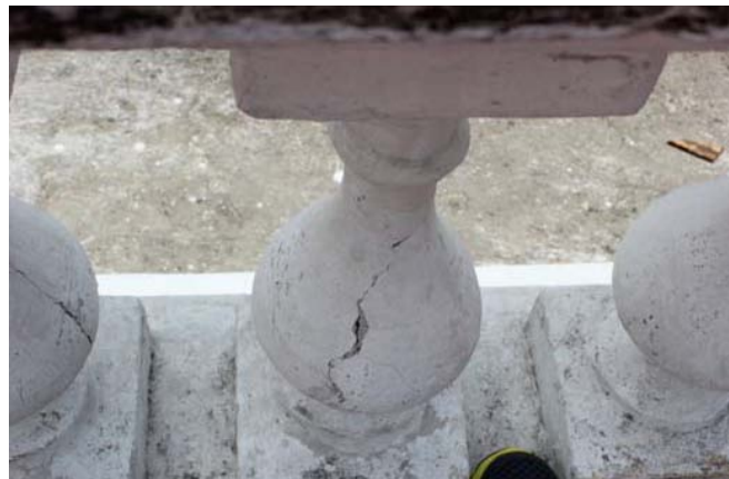
Figure 6: Baluster cracks at the roof parapet
