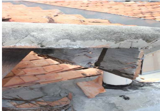
Figure 5: Timber beam decay
