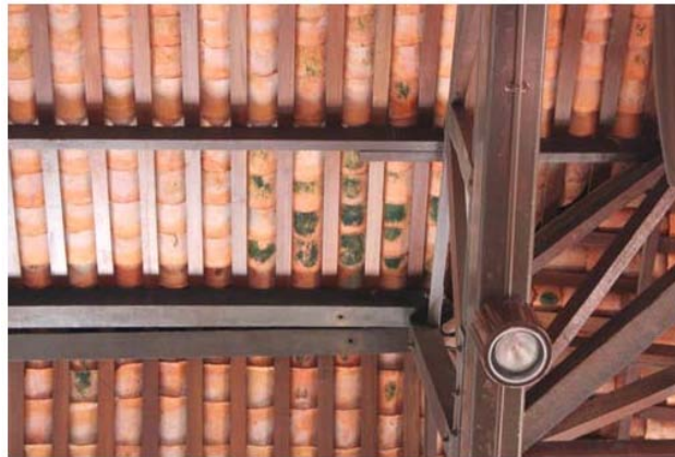
Figure 3: Fungal stains at roof tiles
