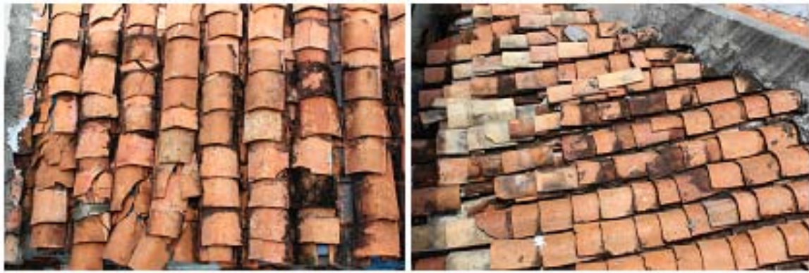
Figure 2: Broken and missing roof tiles
