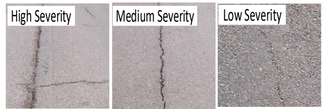
Figure. 11 Examples of different severity levels longitudinal cracks
