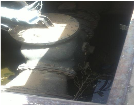
Figure 4: High lift water pump, MWTP
