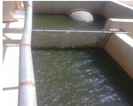
Figure 5: Bar Screen channel, MWTP
