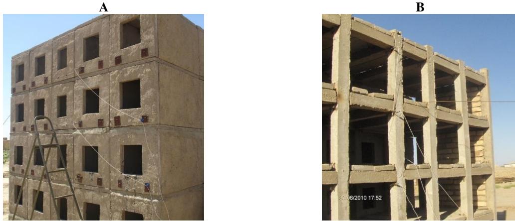
Figure 3 - Model of the section of the building A and model of built stack-like structure B.
