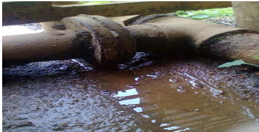
Plate 1. Leakage from the burst pipeline
