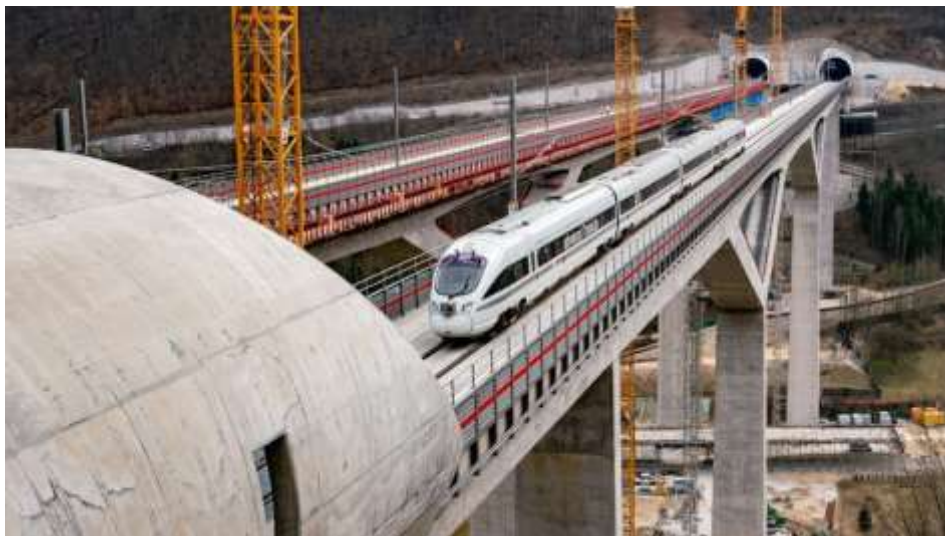
Fig. 13. The first ICE on the Filstal bridge – the highest rail bridge in Baden-Wurttemberg [17] as part of the new railway line between Wendlingen and Ulm [29]
