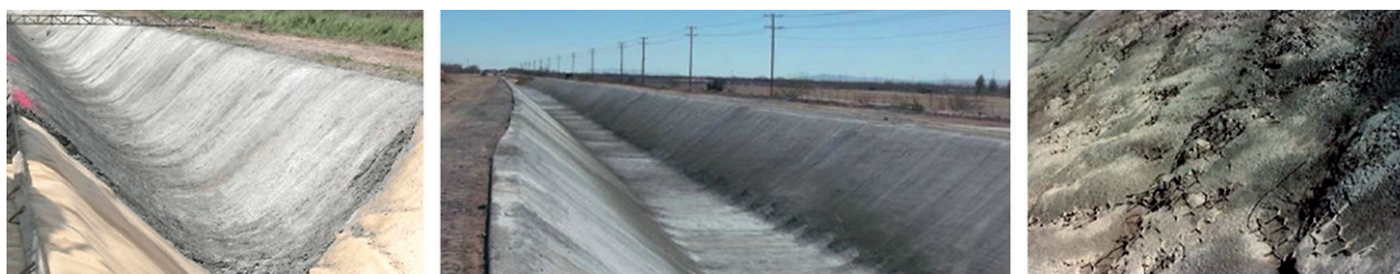
Fig. 1. Pilot sites of irrigation channel lining installation using shotcrete in the south of Kazakhstan
