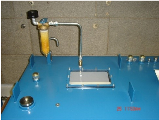
Fig. 3. Operation and appearance of an air dryer (upper), real world example installation on an industrial hydraulic tank (bottom)
