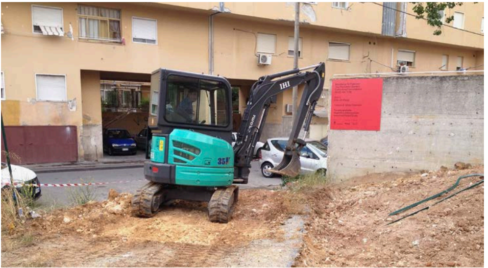
Figure 3. The construction begins during the opening of Manifesta. The first drawing was made directly on site with the excavator, June 2018.
