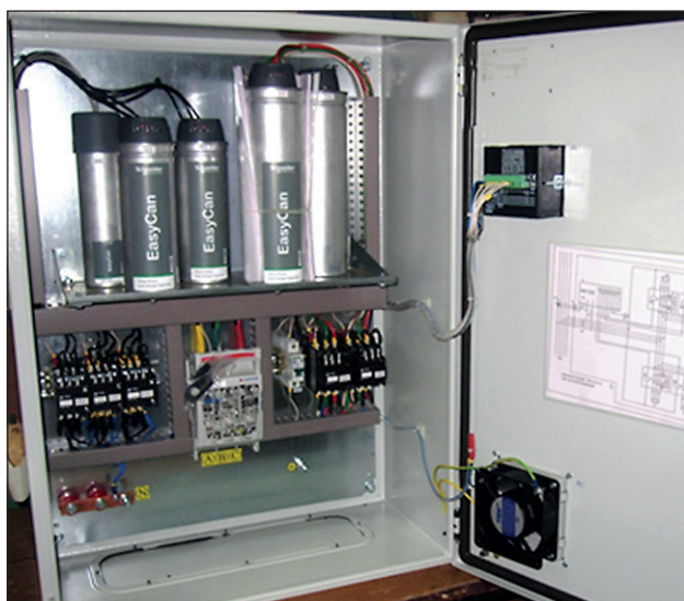
Fig. 9. Capacitor reactive power compensator (CRPC)
