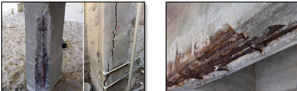
Fig. 3 Damages caused by reinforcement corrosion in columns and beams [16]
