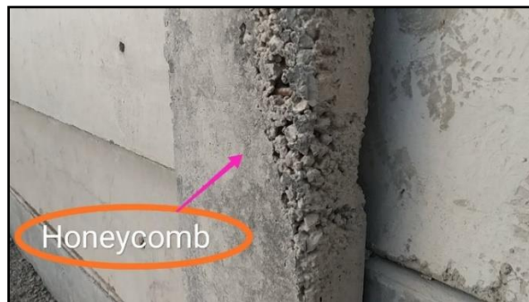
Fig. 5 Insufficient implementation of vibration on concrete pouring [25]
