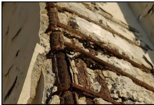
Fig. 6 Inadequate use of concrete cover [27]
