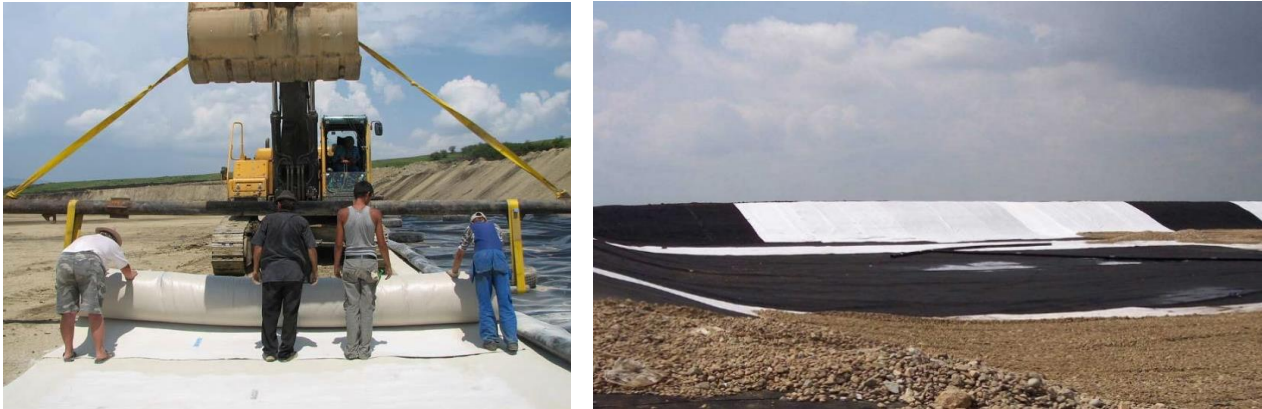
Fig. 1 – Examples of geomembrane and protection geotextile utilisation in the construction of waste landfills
