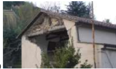
b) Figure 4. Collapses due to wrong interventions, with realization of heavy and rigid concrete curbs not efficiently connected with the roof structure or the masonry walls: a) 2012 Emilia earthquake; b) 2009 Aquila earthquake
