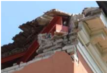
Figure 3. 2012 Emilia earthquake - Collapse due to a wrong intervention, without the realization of an upper curb on the masonry wall to distribute the horizontal forces transmitted by the new steel beams
