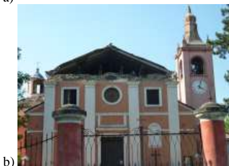
Figure 11. Roof subject to earthquake action in the longitudinal direction: a) scheme of roof forces acting on the pitches; b) collapse of the gable of a church
