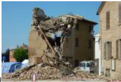
b) Figure 2. 2012 Emilia earthquake - a) collapse due to the absence of connections between floor/roof diaphragms and masonry walls; b) collapse due to the absence of efficient floor and roof diaphragms
