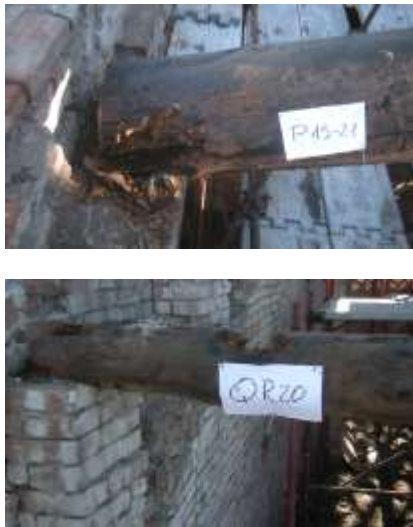
Figure 32. Local damages and deterioration on supports of timber elements.
