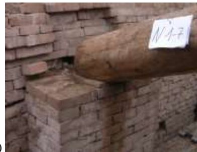
Figure 27. a,b) Relative displacements of diagonal struts of the lateral aisles with respect to masonry support; c) overturning of a masonry wall portion.
