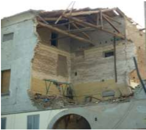
Figure 1. 2012 Emilia earthquake - Collapse of external slender walls due to the absence of the intermediate floor and insufficient stiffness at the roof level.
