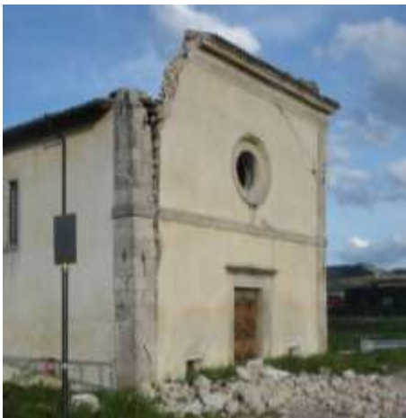
Figure 6. 2009 L'Aquila earthquake - wall detachment due to the absence of a roof structure capable of ensuring a box-like behavior of the church
