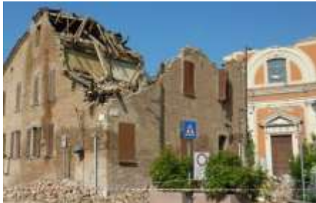
Figure 5. 2012 Emilia earthquake - collapse due to unbalanced horizontal thrusts of roof structures
