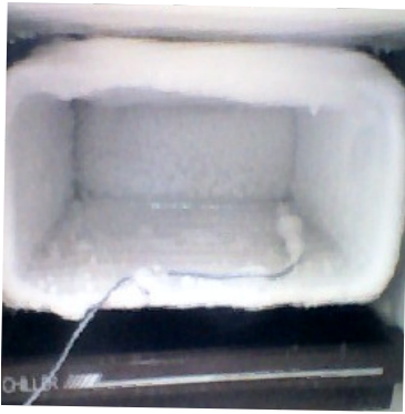
Figure 6 : Formation of ice on chillier without coating in the experiment with 20litres of water load run for 25 hrs.
