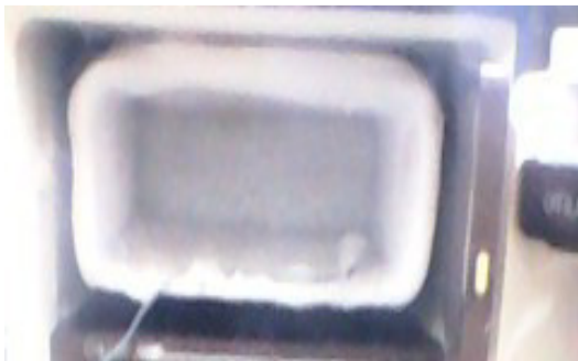
Figure 8: Formation of ice on chillier without coating in the experiment with 20litres of water load run for 50 hrs.
