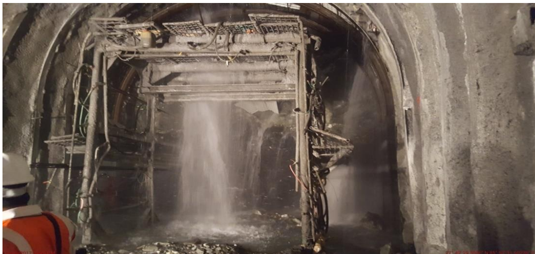
Plate 4.3: See page water coming from crown part of tunnel
