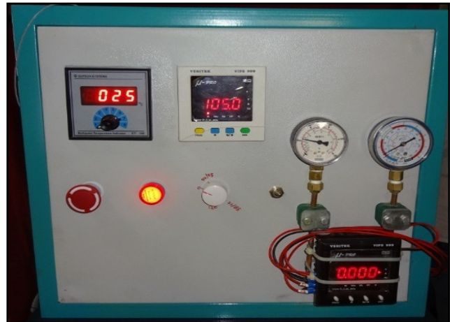
Figure 2.2: Control panel of system
